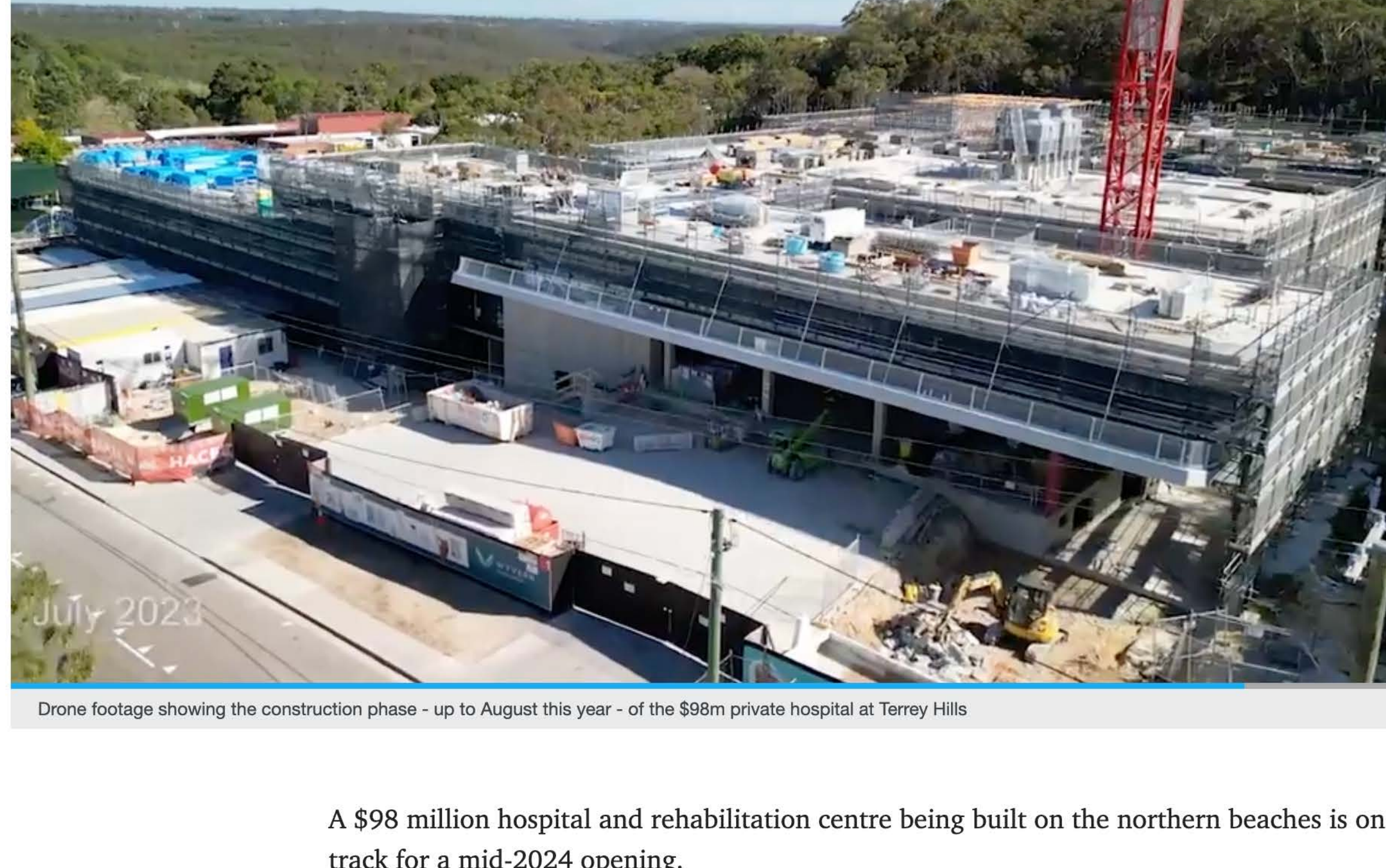
Drone footage showing the construction phase - up to August this year - of the $98m private hospital at Terrey Hills
