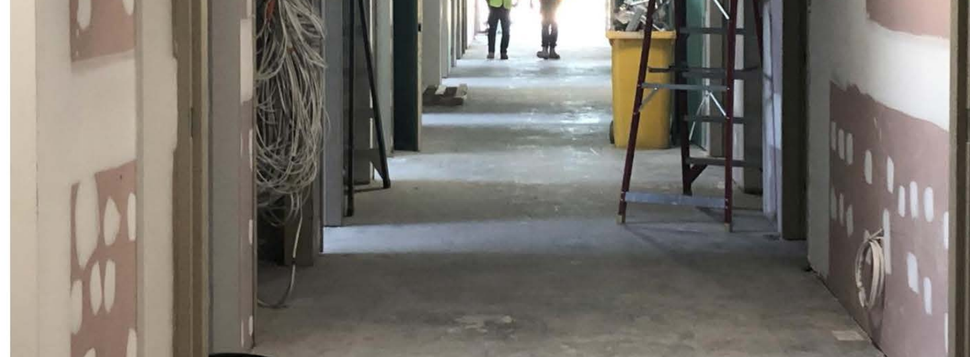
Construction workers in the building accommodating the general and surgical wards at the hospital. Picture: Jim O'Rourke
