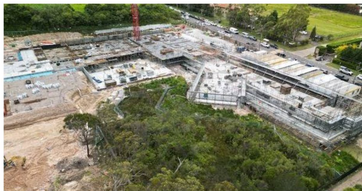
Excavation works have been completed at the Wyvern site and construction is under way
